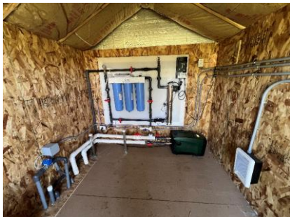
Filter and treatment board.
