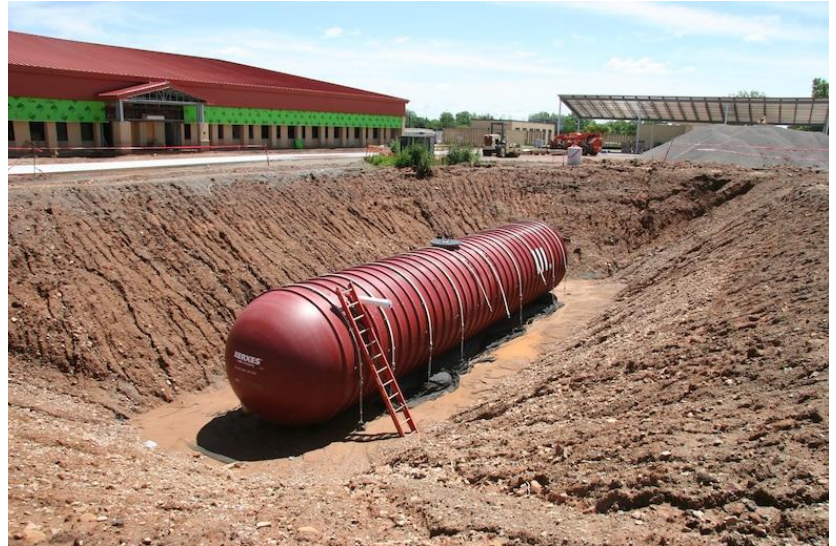
The 30-thousand-gallon rainwater collection tank at the Reception Complex under construction at Fort Sill.
