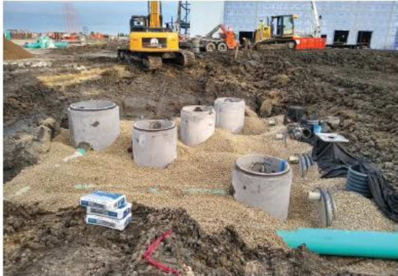
Installation of the system. The ends of the buried storage tanks can be seen on the right.
