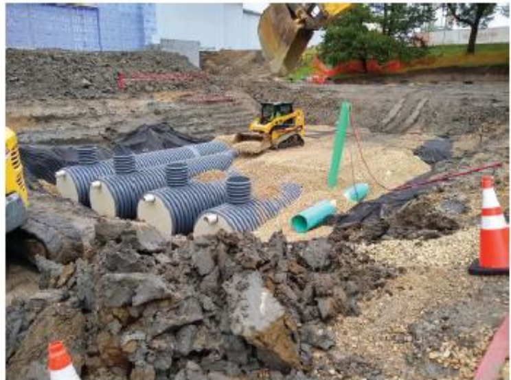
The four underground storage tanks can hold a combined total of 52,000 gallons of rainwater.
