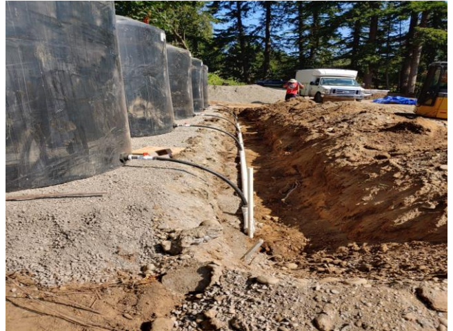
Water storage tanks with manifold.
