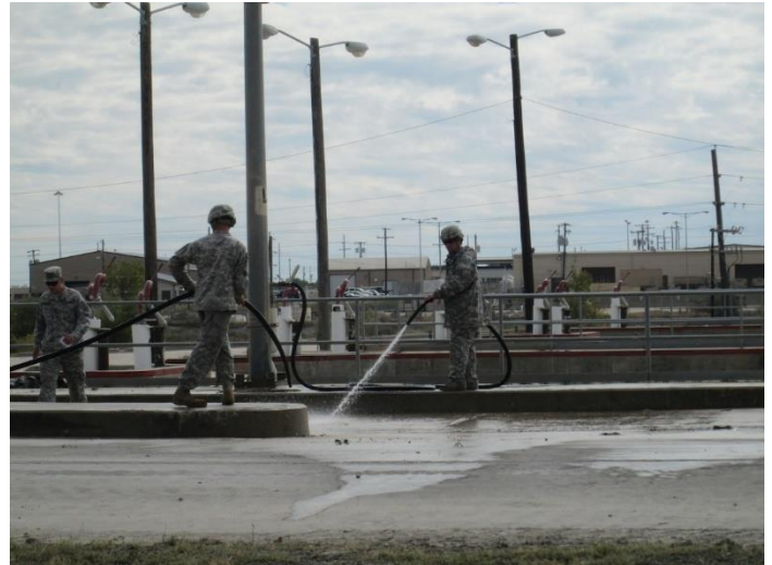
Fort Hood's Tactical Vehicle Wash Rack captures rainwater for use and also treats off-wash for reuse
