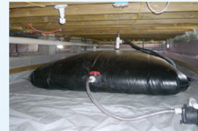
New Orleans, LA. 1,000-gallon pillow installed under home in horizontal, wasted space; www.rainwaterpillow.com ; submitted by Jim Harrington.
