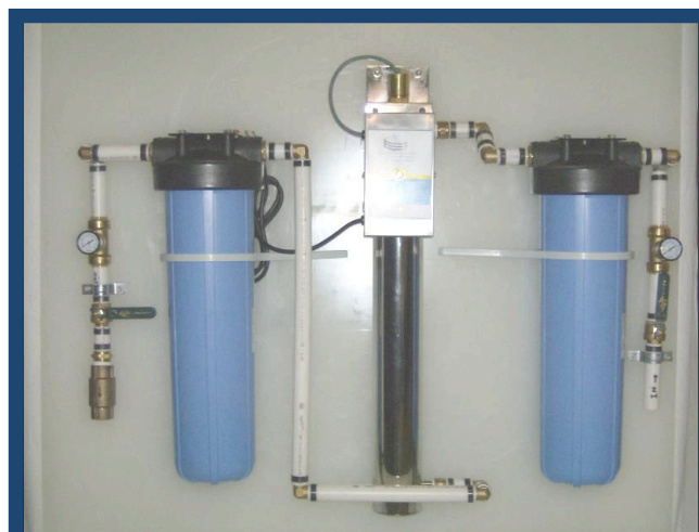
Figure 16. Water treatment system using a sediment filter, an ultraviolet light and a carbon filter.
